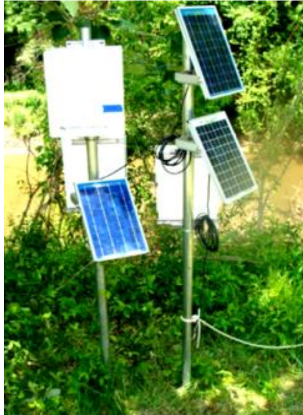
Figure 6.3 Data loggers and solar panels attached to a pole on the nearby floodplain.
